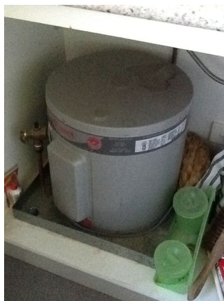
Photograph 20: Staff room water boiler
