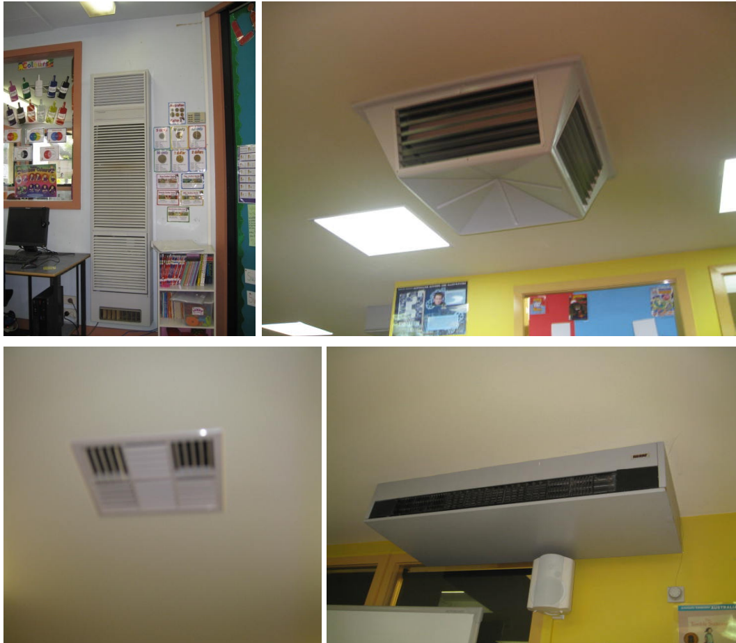
Photograph 10: Heating and cooling systems.
