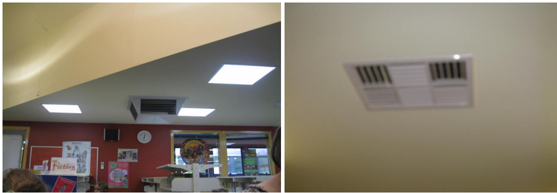
photograph 15: Evaporative units and ducting.
