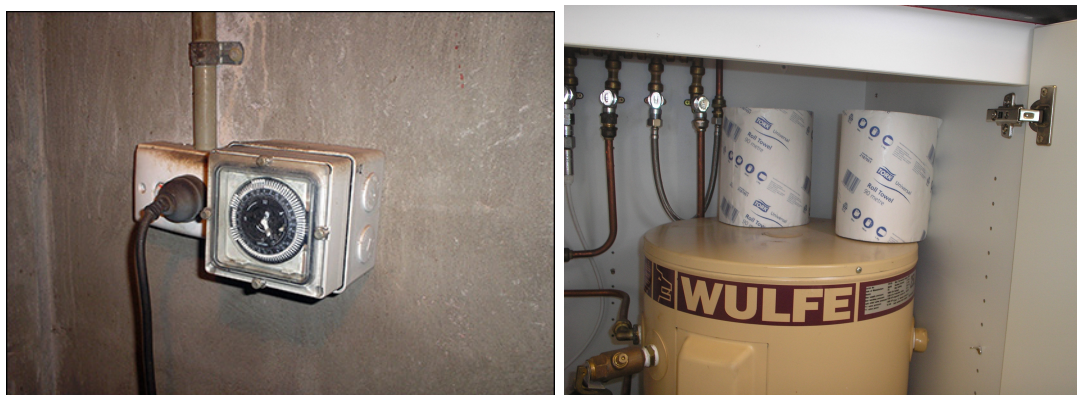
Photograph 21: 365-day hard-wired timer for hot water services.
