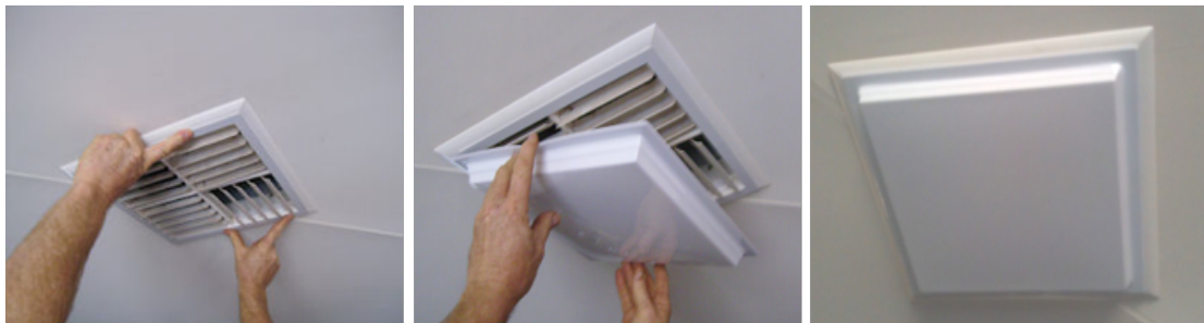
photograph 16: Winter covers for ducted vents
